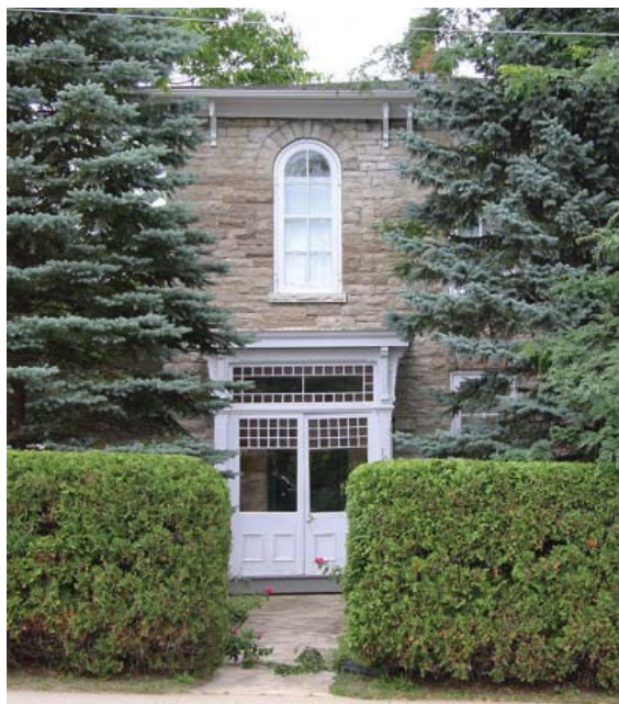
Example of a well-maintained entry vestibule. Other decorative wood elements include the arched window, and cornice brackets, as seen at the Doctor's House on Queen Street.
