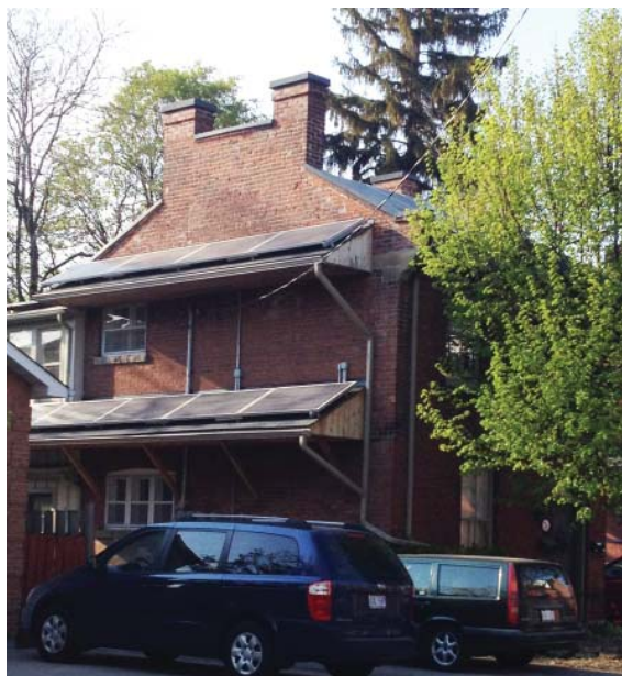
Solar collectors installed on the rear elevation of a house.
